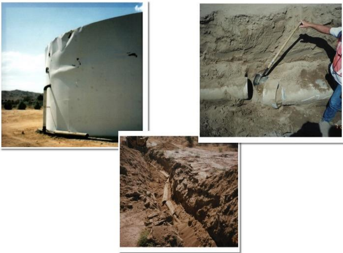
Figure 3 Examples of Earthquake Damage to Water Facilities in the 1992 Landers Earthquake
