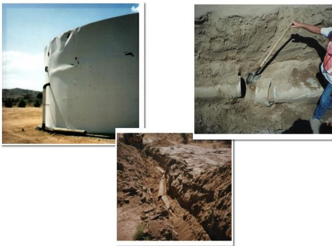
Figure 4. Examples of Earthquake Damage to Water Facilities in the 1992 Landers Earthquake. * Pictures above are from Hi-Desert WD and Bighorn Desert View Water Agencies.
