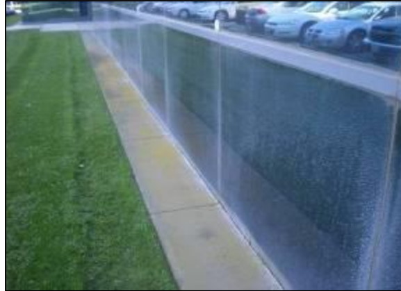
Water Spots on Windows
