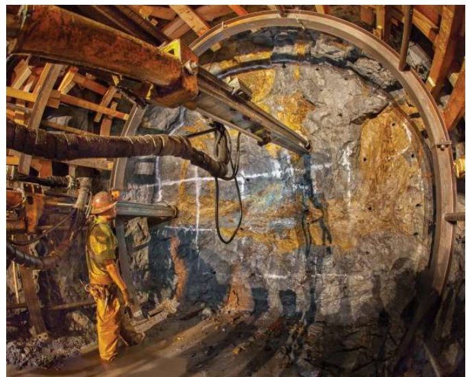
Above: Tunnel junction with construction shaft. Below: Drill and blast method was used to excavate tunnel.
