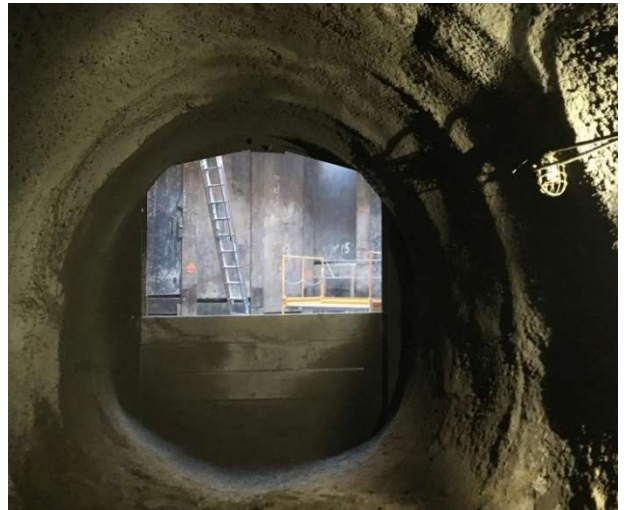
Figure 9. SEM Tunneling for City Trunk Line South Across Tujunga Wash - AECOM and DSP jointly designed the SEM tunnel along an S-shaped alignment.
