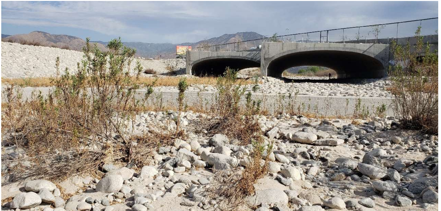
View of City Creek, looking upstream at the Alabama Street bridge crossing (part of the Wash Plan HCP).
