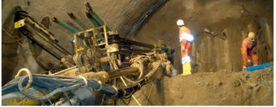
Figure 9. In-tunnel dewatering system.
