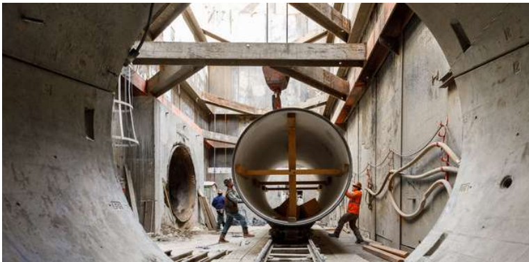
Pipe section from image above now lowered into place in the tunnel at RSC Units 5 & 6.
